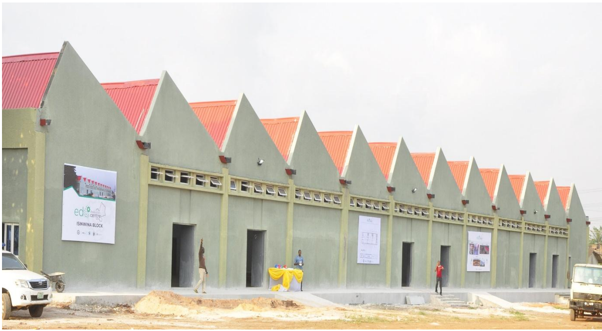
EDO STATE PRODUCTION CENTRE AT OLD PRINTING PRESS PREMISES, SAPELE ROAD, BENIN CITY
